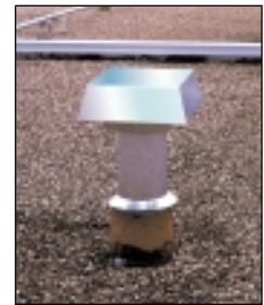
roof mounted hood
